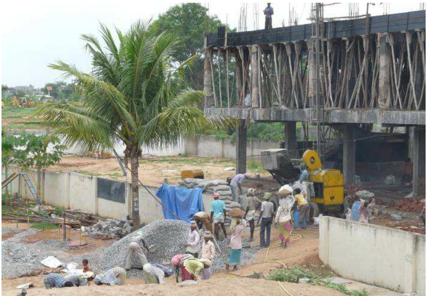
Hyderabad , photo of the new building taken from the roof of the old, showing the far wall, which encloses the additional land purchased for the new building. We'll tear down the wall between the two when construction is finished. Johanne photo.
